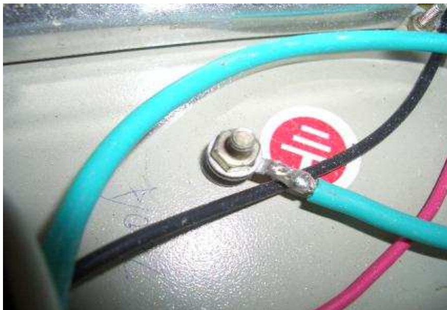
Photo 21 - Earthing terminal in the main control box
