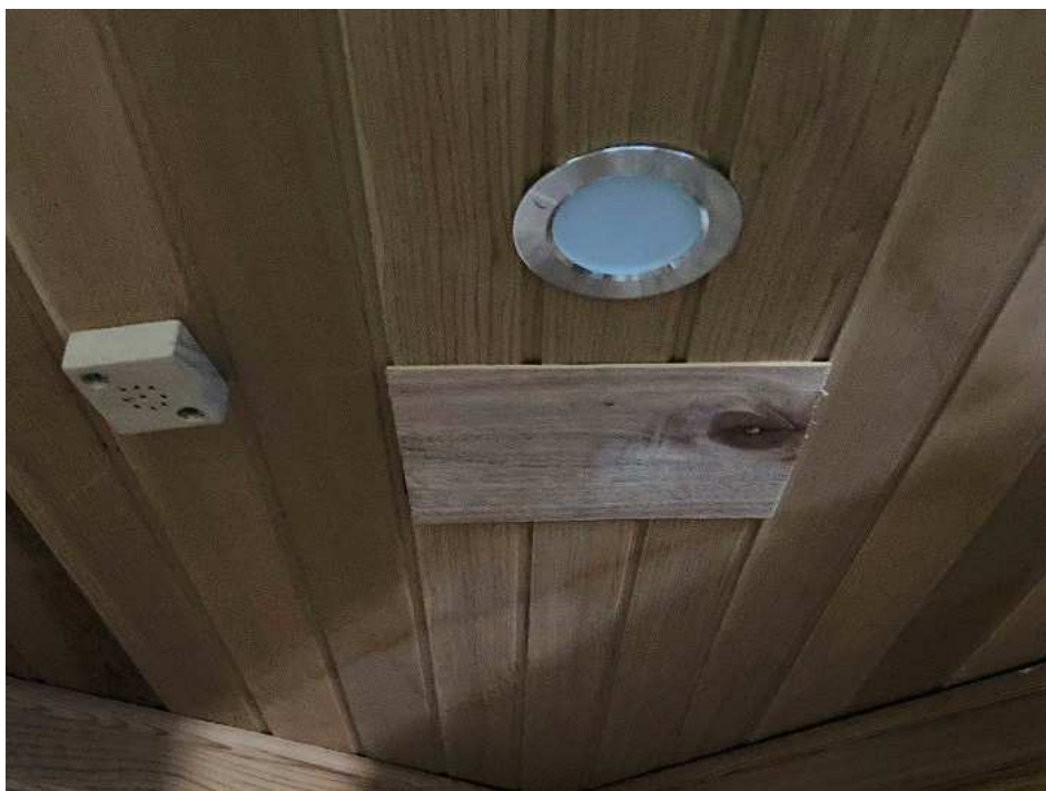
Photo 5 - Internal lamp on the ceiling
