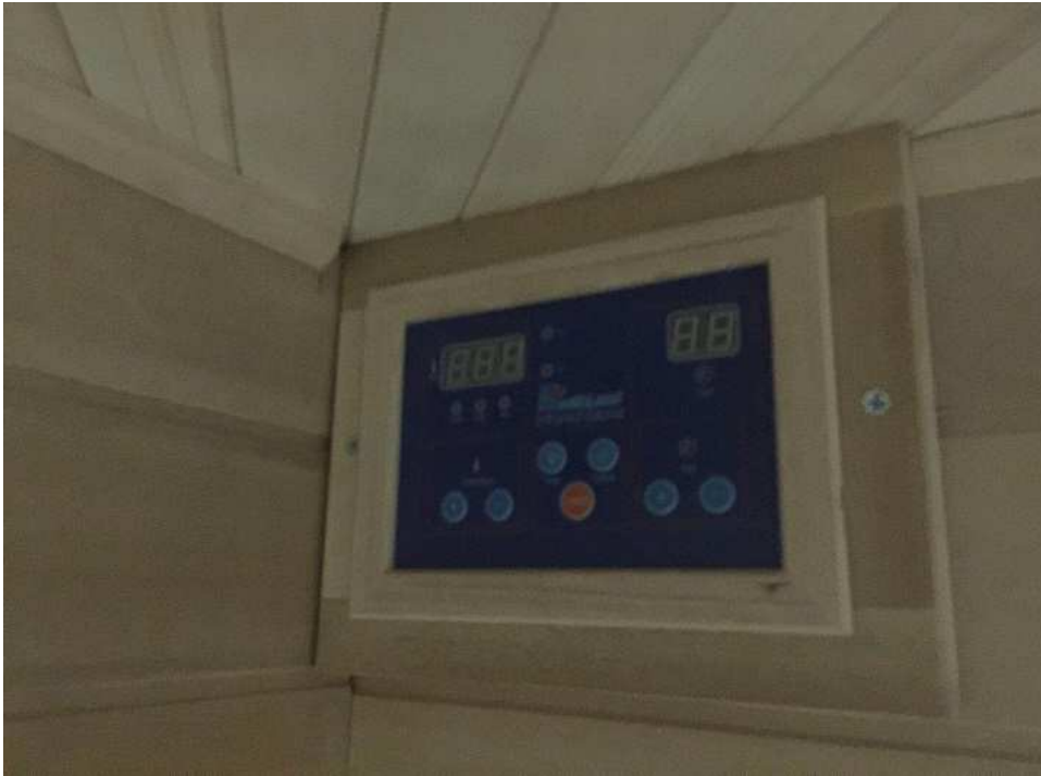
Photo 11 - Internal control panel
