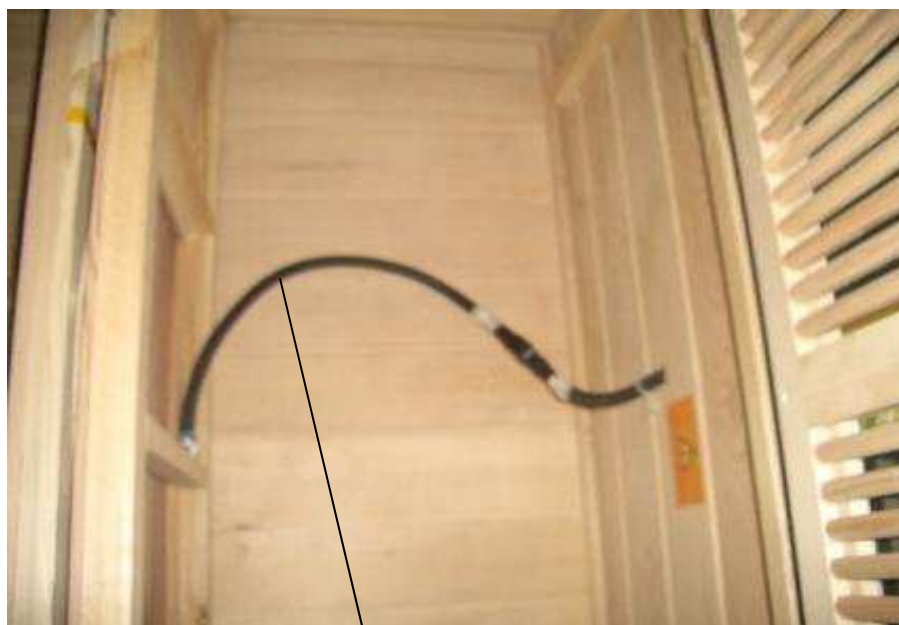
Photo 16 - Cord and Connection under seat, which cannot be contact without aid of tool, the interconnection cord is enclosed by metal conduit
