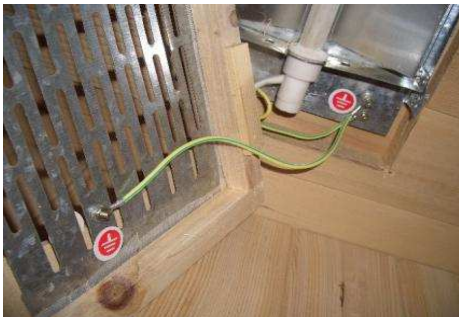
Photo 14 - Earthing mark (Note: The insulated tape cover the metal guard of the heater)
