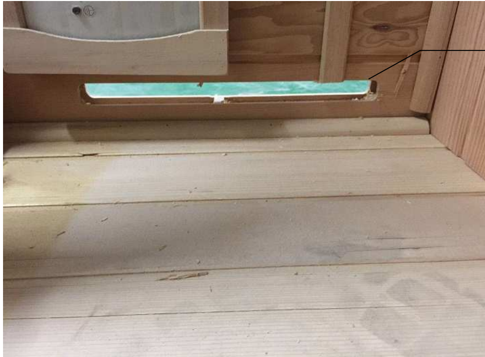
Photo 6 - Inlet ventilation (HL-200A)
