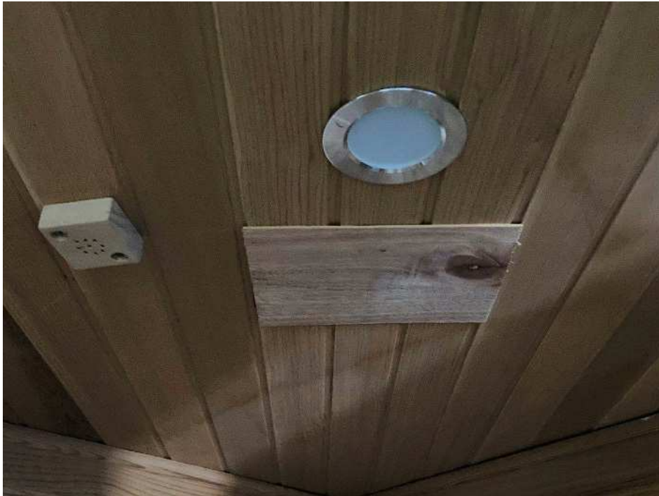
Photo 5 - Internal lamp and wood guarded temperature sensor on the ceiling
