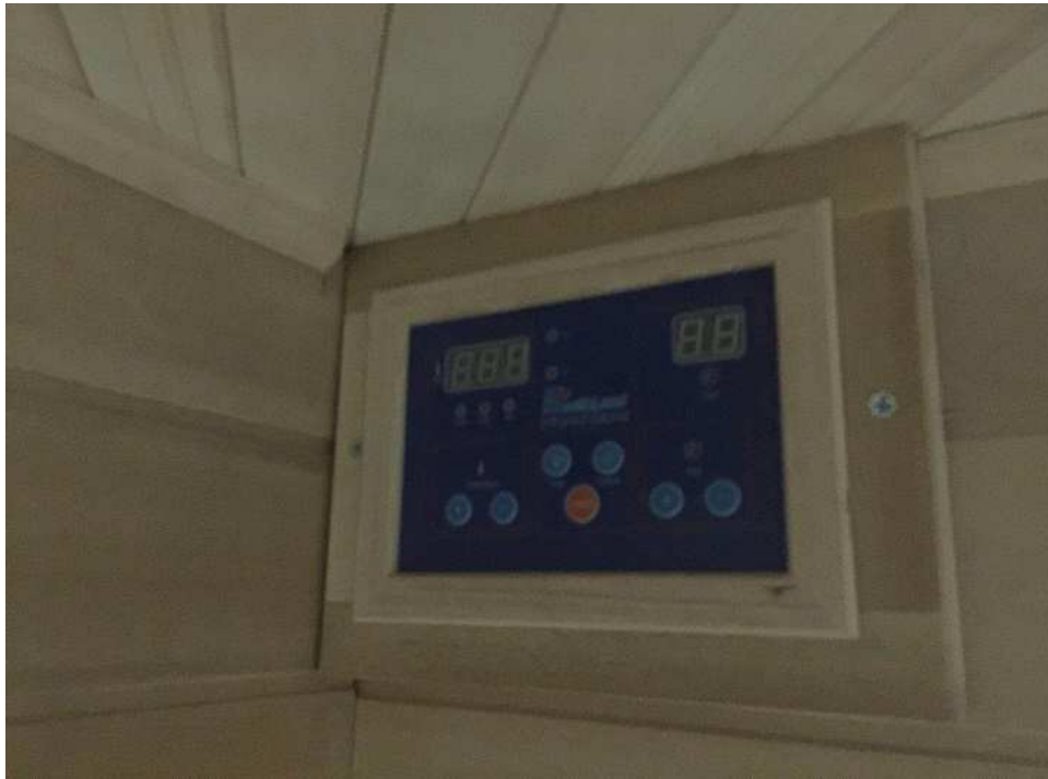
Photo 11 - Internal control panel
