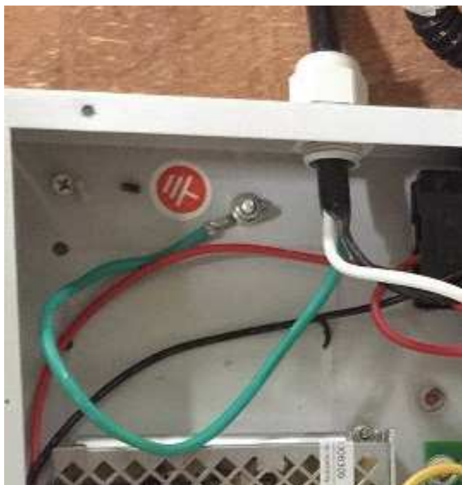
Photo 13 - Protective bonding terminal in control box
